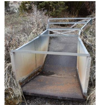
Measurement flume needing replacement Photo. Phil Brink
